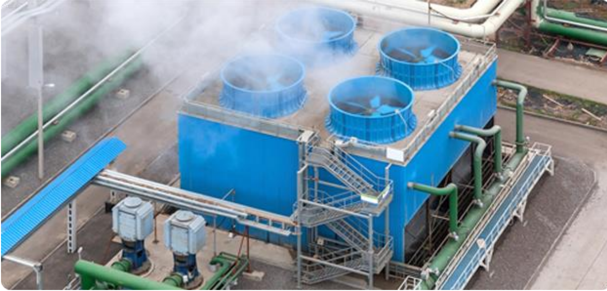
Water cooling towers
