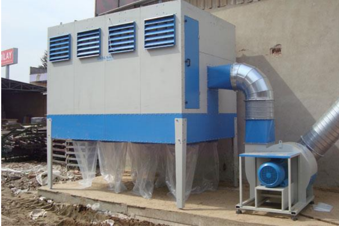
Dust Collector System
